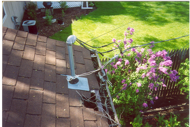
A family of three raccoons made themselves at home in the attic of this house. The hole in this roof was the entry point. Please also note that the temporary repair to the electrical service is not the safest.
